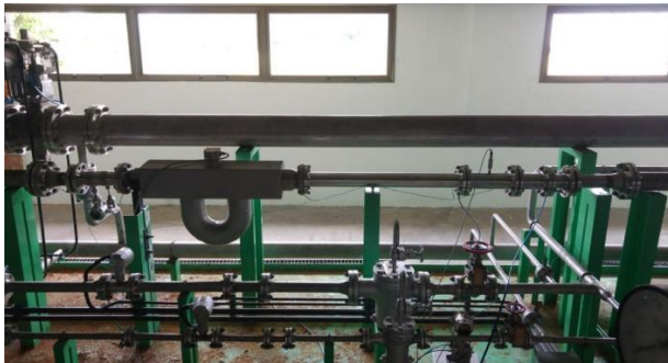
Installed MUT during comparison calibration
