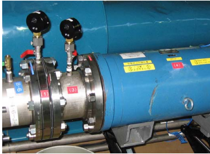
Fig. A1-16 Pressure measurement at the two pressure taps of the upstream pipe with the filter if necessary.
