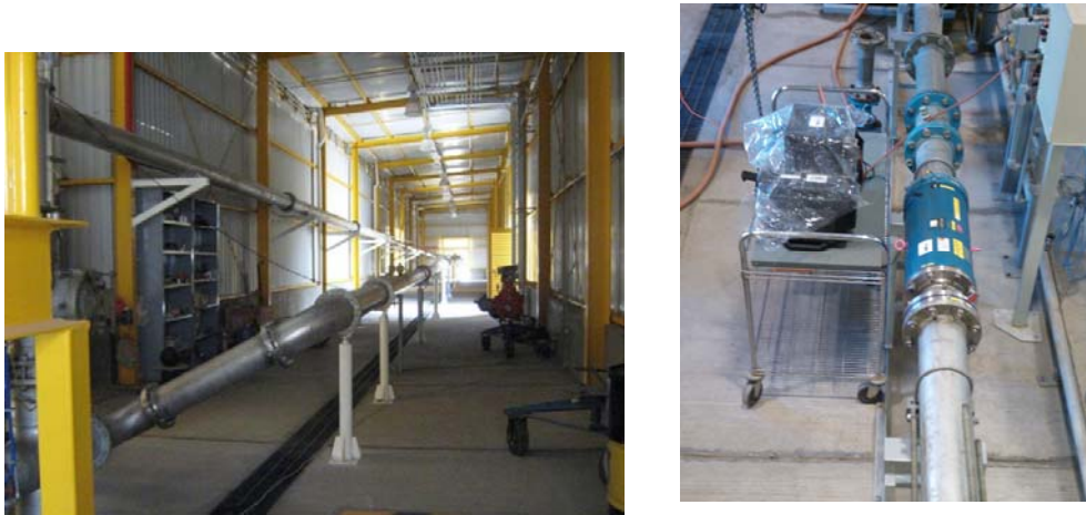
Figure B-2-1 a) Images of the reference system at CENAM, b) installation of the K2 TS at CENAM.
