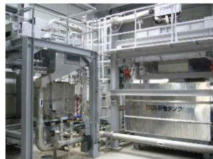
Weighing tank (5t)
