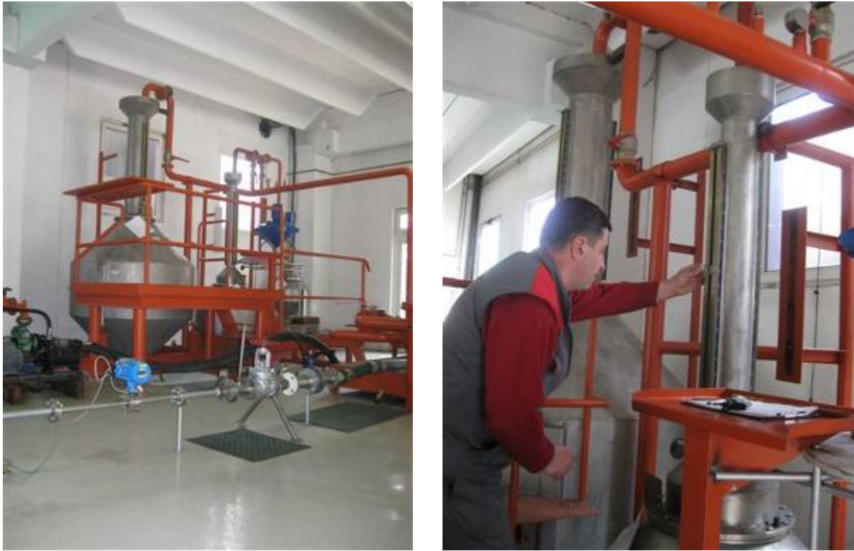
Fig.5.14 The facility of IMBH.
