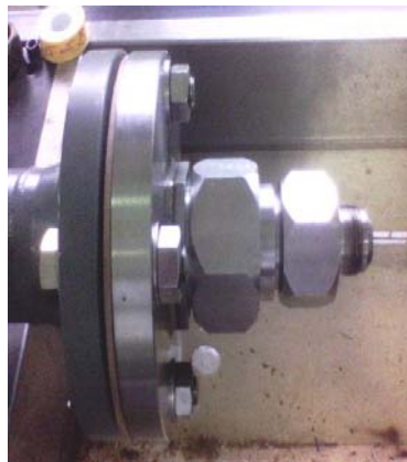
Fig 10. Reducer Pipe as Protector of Mechanical Seal in the Flange
