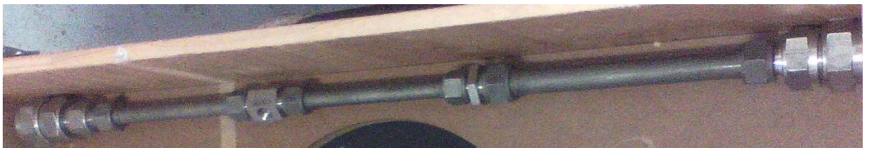
Figure 2. FT-12 (Meter 1) with Adapter and Reducer Pipe
