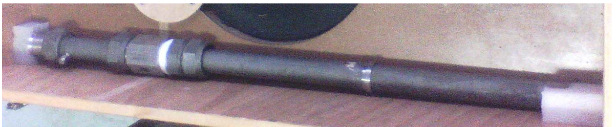
Figure 3. FT-24 (Meter 2) with Adapter and Reducer Pipe
