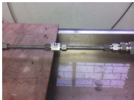
Fig 15. FT-12 Fully installed
