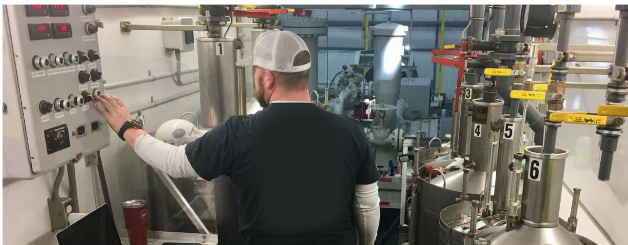
Figure 1. A metrology technician at a crude oil pipeline location uses NIST-calibrated volume test measures to calibrate industry “provers” that are then used to calibrate pipeline flow meters. This includes test measures of 100 gallons (1 and 2 on the upper left) and 50, 25, 10, and 5 gallons (3, 4, 5, and 6 on the right, respectively).
